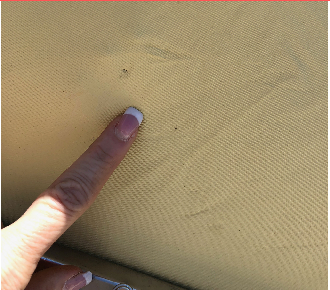
1st TOP INSTALLED DRIVERS SIDE DAMAGE - INTERIOR DAMAGE EVIDENT COMPRESSION DAMAGE CAUSED BY FRAME MISALIGNMENT WHILE FOLDING DOWN
