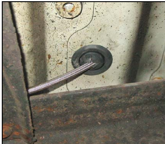
Figure 12 Floor access hole
