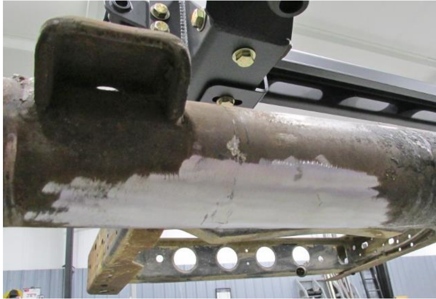
Figure 21 – Cut Off Factory Lower Shock Mount (Passenger Side)
