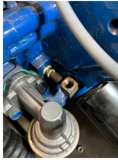
1/4" NPT extension pipe with 90 degree fitting installed.
