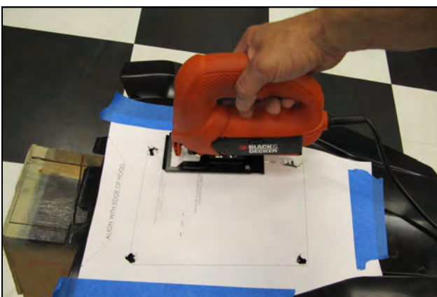
37. Using a jigsaw or equivalent, cut along the template line and connect the 1/2" holes. Remove the hood center, Template and tape.
